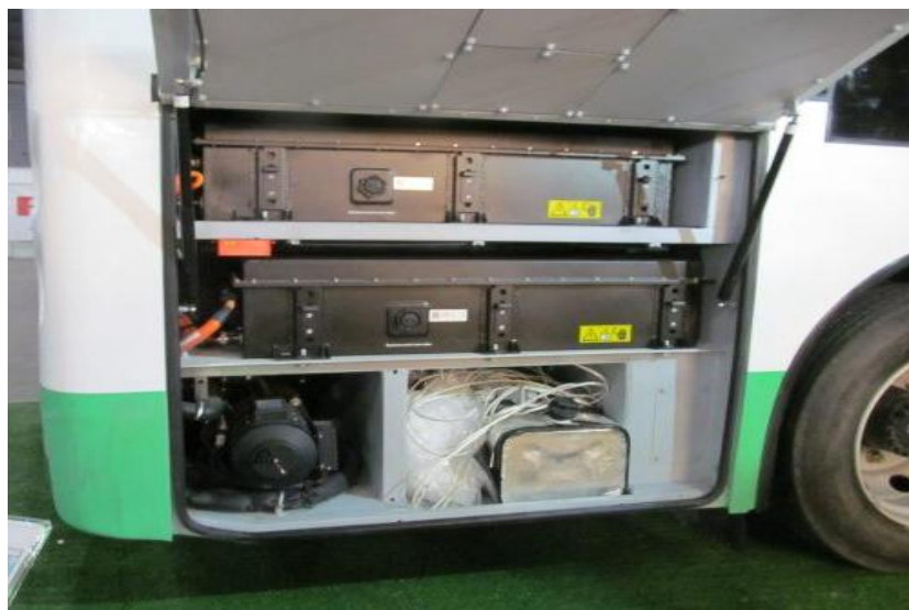
Figure 2 – Electric bus battery compartment
