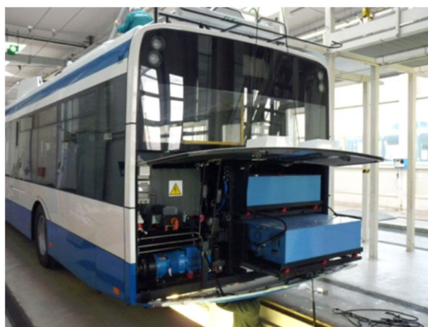
Fig. 3 Traction NiCd batteries (right) and DC converter (left)
