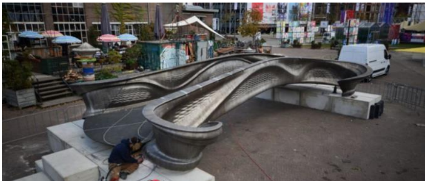
Fig. 12. A stainless-steel bridge construction, made with the use of an automated 3D print technology
